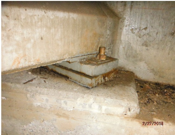
Photo 3. LBP Positive Beam Bearing Plate
