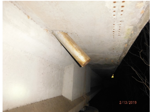
Photo 4. LBP Positive Drainage Scupper
